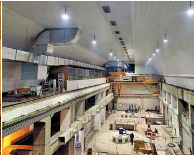
Machine Hall at 60 MW Naitwar Mori HEP, Uttarkashi, Uttarakhand.
