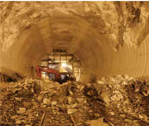
Niche Excavation Work in Progress at Alimineti Madhva Reddy, Irrigation Tunnel, Andhra Pradesh.
